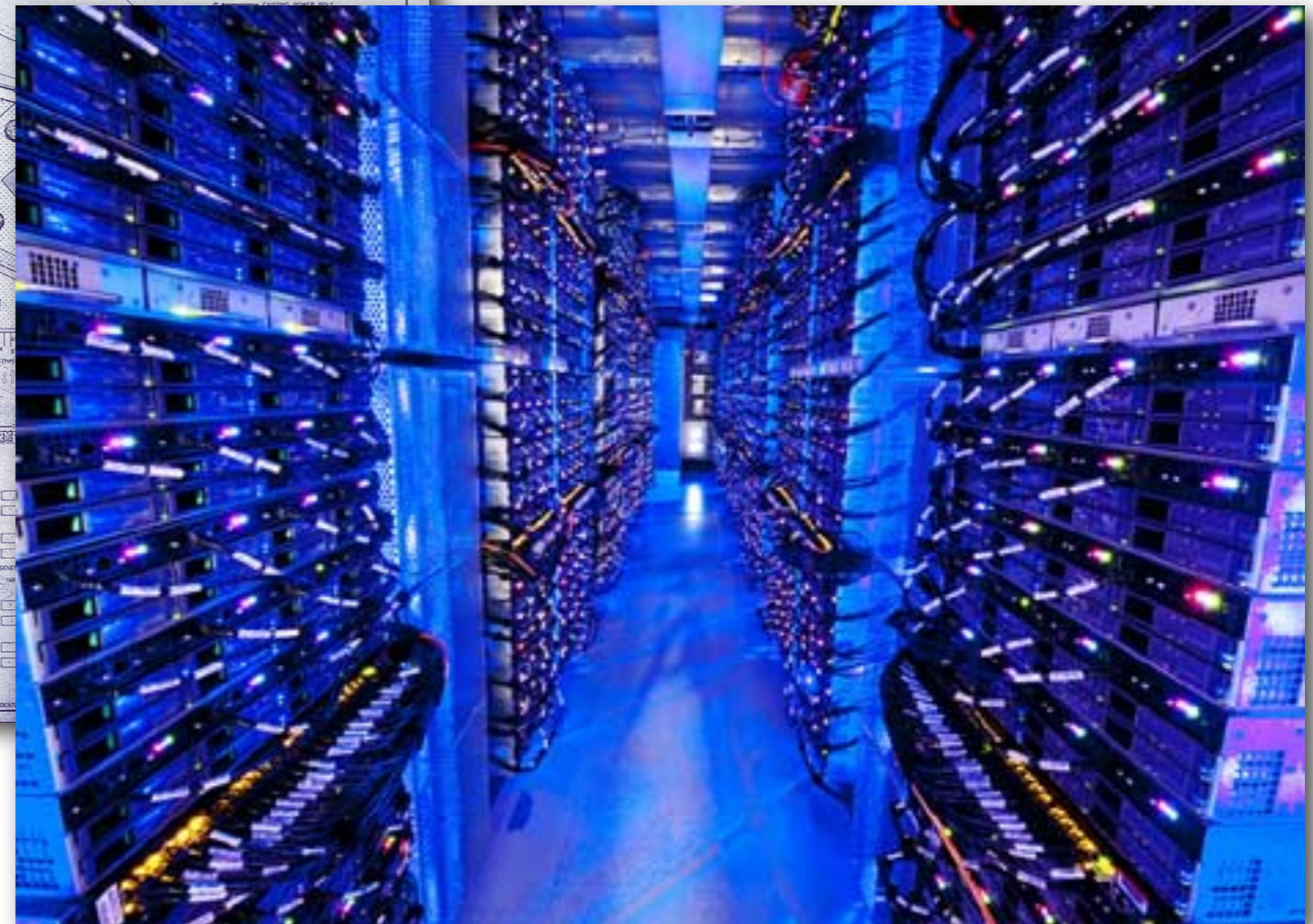
A 40-foot container inside the new Microsoft Chicago data center http://www.forbes.com/forbes/2009/1116/outfront-ibm-cloud-microsoft-new-cloud-computing.html
